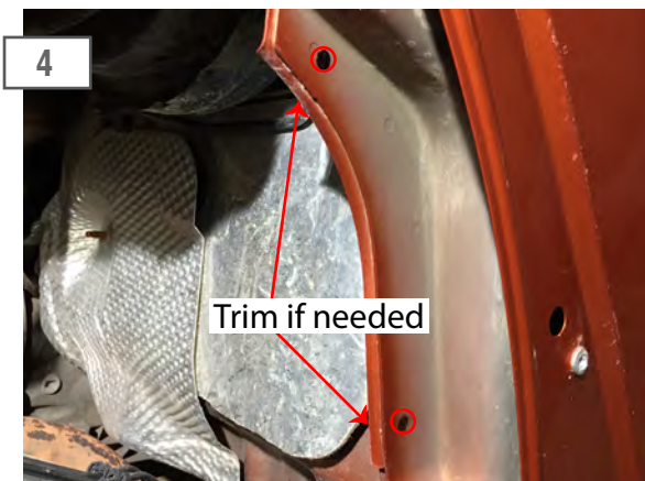
4 Drill a 1/8" pilot hole and then drill the holes to 3/8". Install the supplied clip nuts. **Note: It may be necessary to trim the inner fender lip in order to slide the clip nut on.
